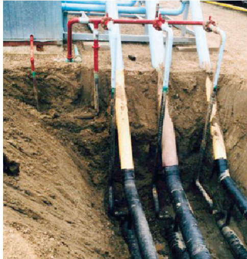
Live Gas Lines Exposed
